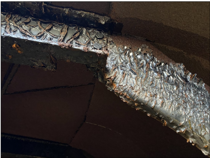
Photo 44 – Failed coating and corrosion at rafter
