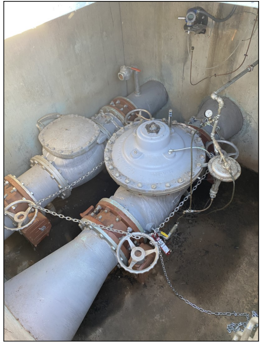
Photo 6 – Inlet/Outlet piping altitude and check valves
