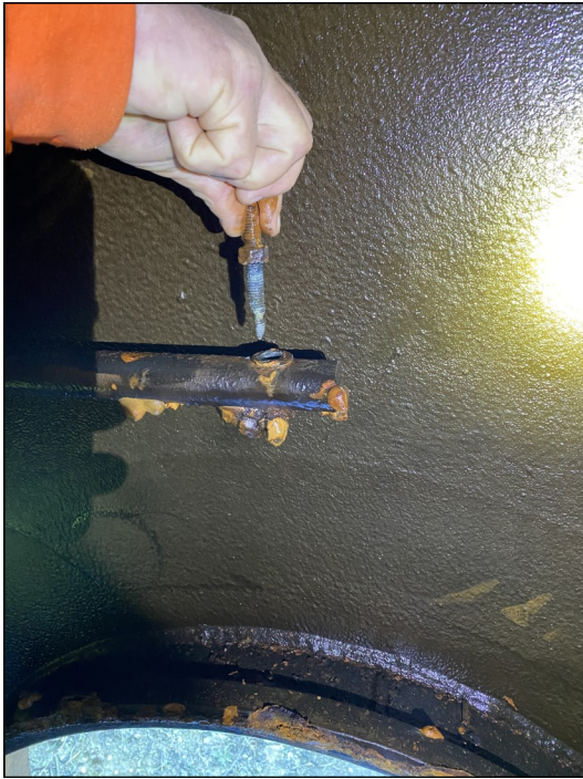
Photo 29 – Corroded bolt at interior manway support
