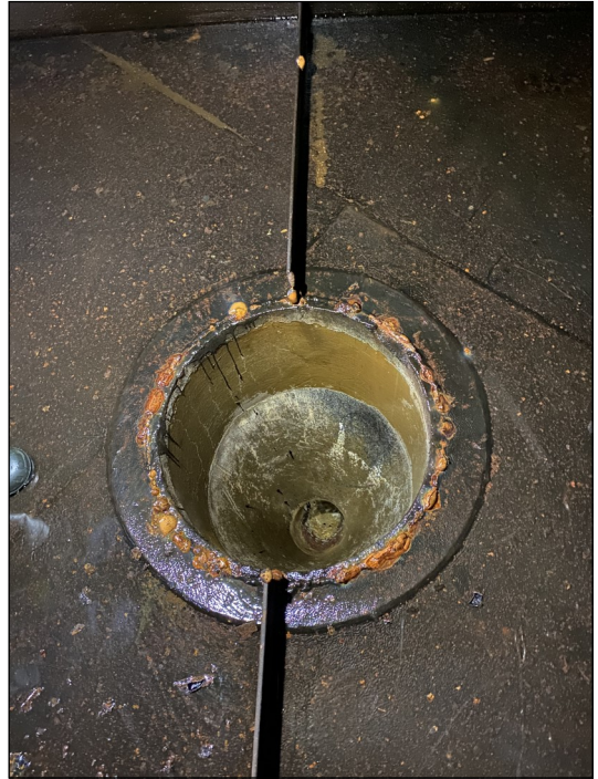
Photo 26 – Tank drain outlet
