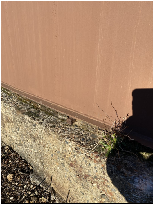
Photo 5 – Exposed tank footing
