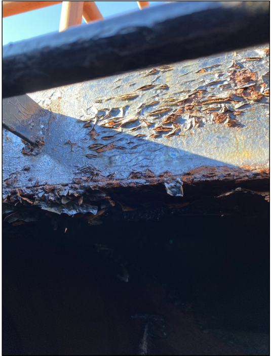
Photo 42 – Failed coating and corrosion at rafter near roof hatch
