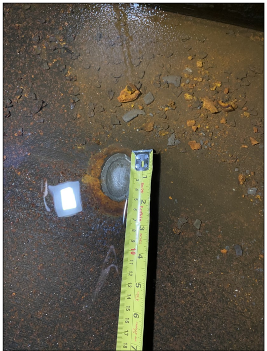
Photo 28 – Tank floor corrosion pit
