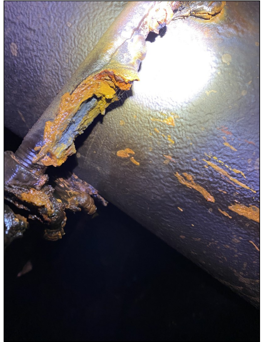
Photo 30 – Corrosion at interior manway support
