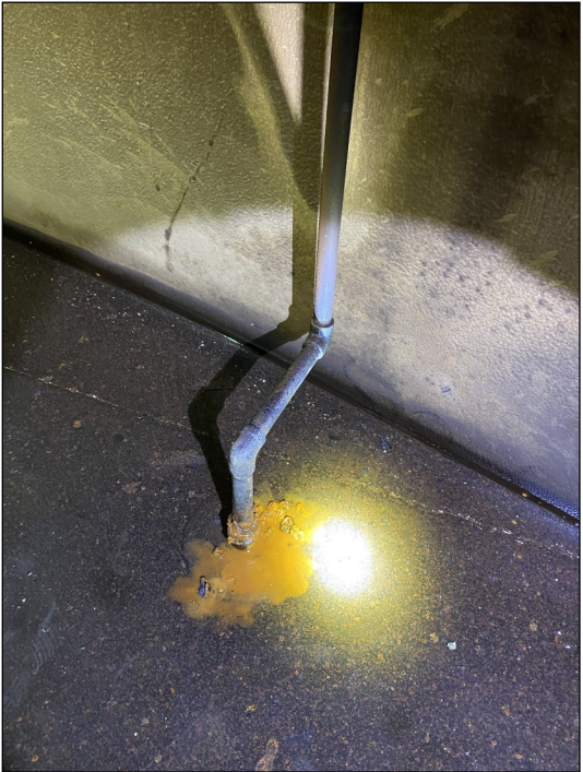
Photo 24 – Altitude valve control piping
