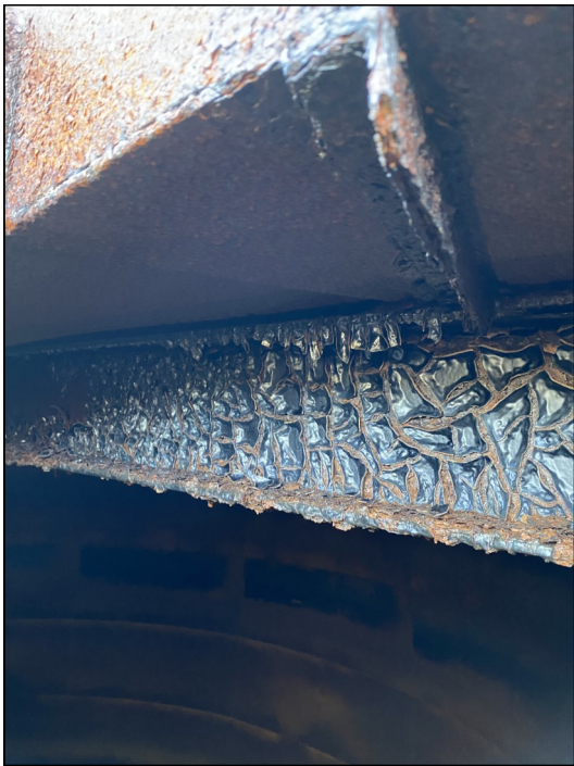
Photo 43 – Failed coating and corrosion at rafter
