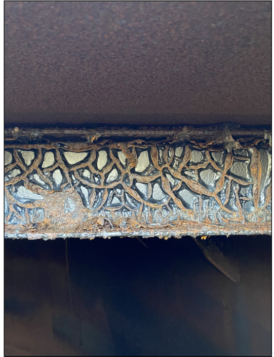
Photo 38 – Failed coating and corrosion at rafter
