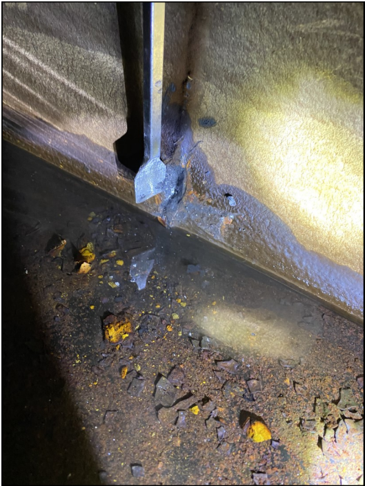
Photo 23 – Corrosion pitting at wall plate weld seam
