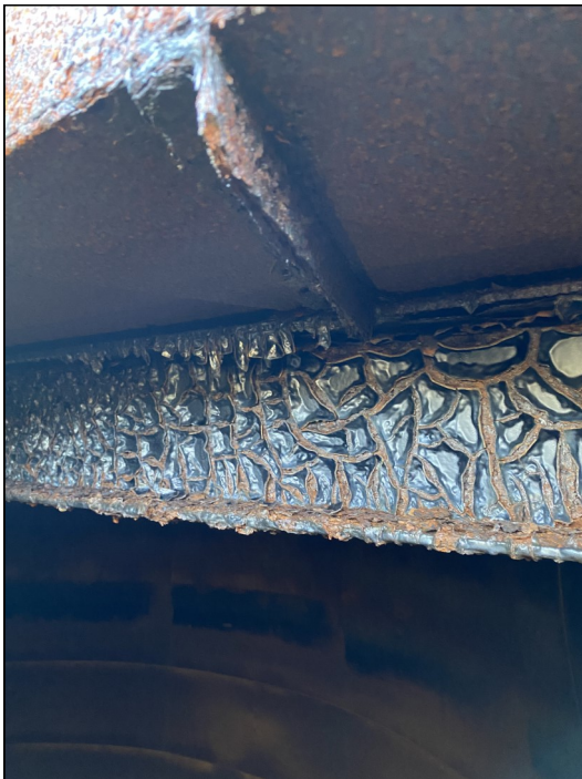
Photo 39 – Failed coating and corrosion at rafter
