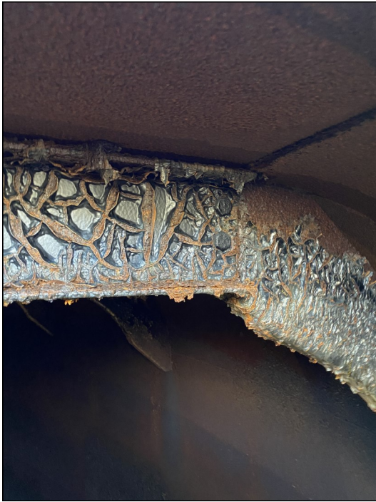
Photo 41 – Failed coating and corrosion at rafter
