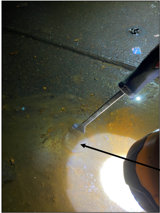
Photo 21 – Tank floor corrosion pit
