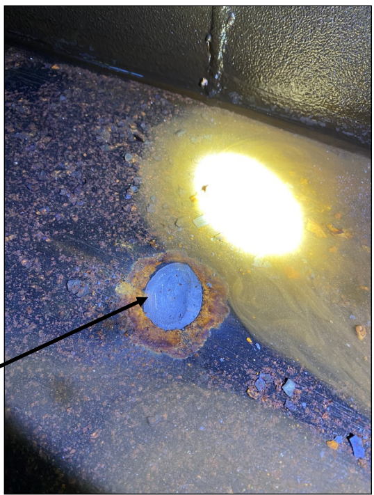
Photo 12 – Tank floor corrosion pit
